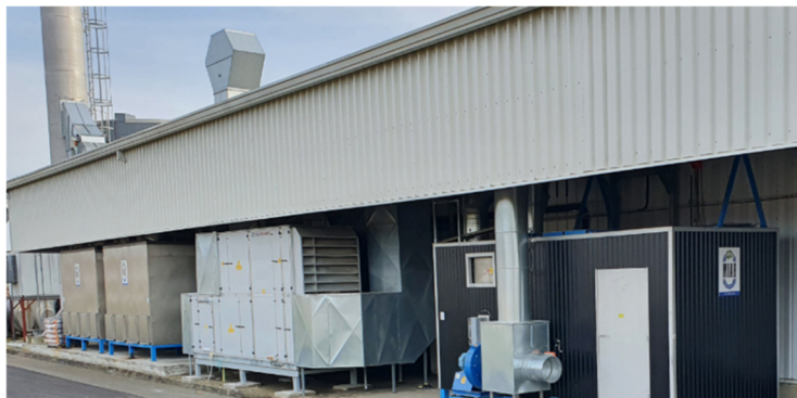
Photo 1. MIAB FD system with two filters, see two stainless steel units to the left, as well as the catalytic oxidization unit, see black unit with a door to the right.
